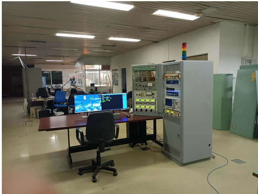
Figure 40: The new computerized control
